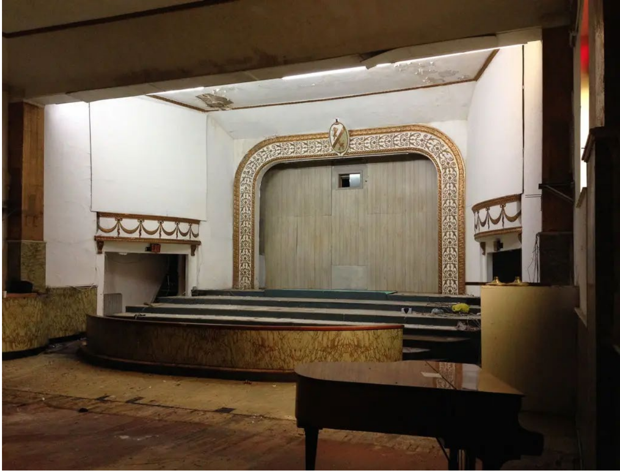
The proscenium arch at the Child's Memorial Temple Church of God in Christ, a remnant of the Harlem building's days as a theater. Photo: David W. Dunlap/The New York Times
